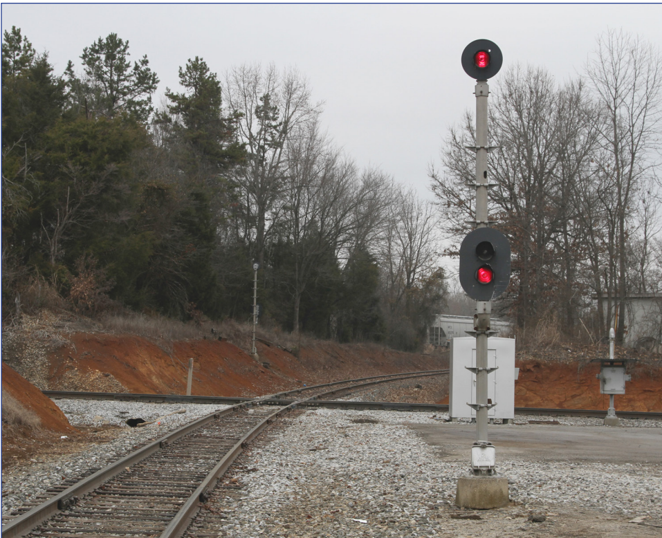
Present day Barber Junction. The upper image is looking west along the Norfolk Southern mainline; the lower shot is looking north along the old line to Mocksville. Note the signals protecting the main line and the phone box.
