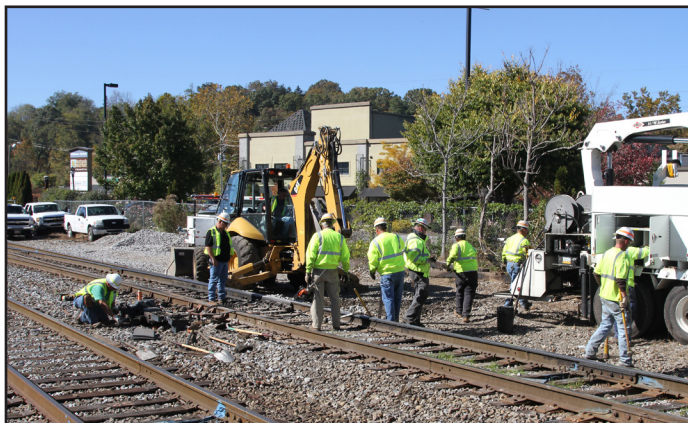
On October 23, a Norfolk Southern track crew was working on a turnout in the Biltmore yard in Asheville.
